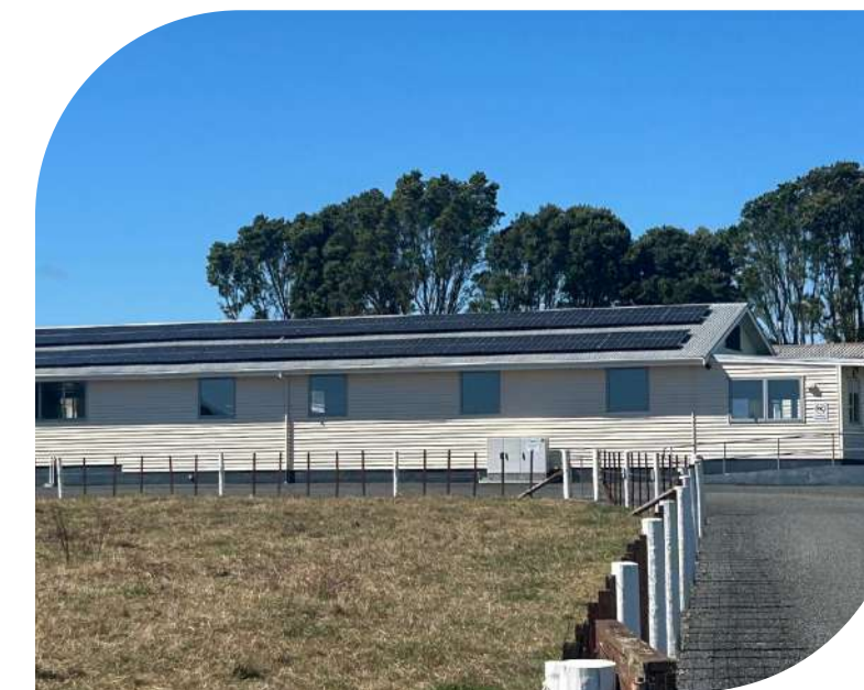
Above: Todd has covered 50% of the costs for an 80 kW solar and battery system at Taranaki's Urenui Marae (Ngāti Mutanga, Urenui Pā Trust) which now provides all electricity for the marae and an electricity export revenue stream.
